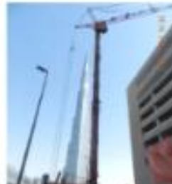
2013 Chiller lift Downtown
