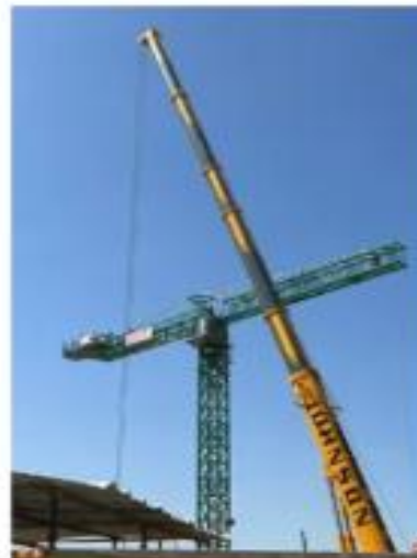
Ras Al khor, Dubai This project was to set up Jaso cranes for a project.
