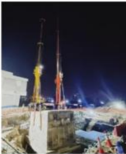
Meydan Site, Dubai Lifting & Re-locating of precast chamber 132tonnes using a 700t and a 500t mobile crane for tandem lift.
